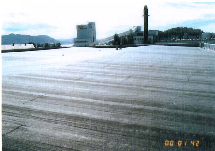
Photo 30: Example of excellent roofing (from T10).
